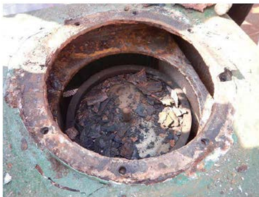
Excess Corrosion of inside of air pipe head
