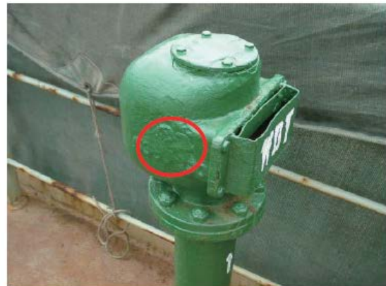
Inappropriate temporary repaired by putty
