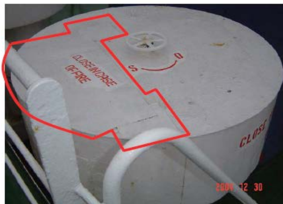
Inappropriate temporary repair by tape
