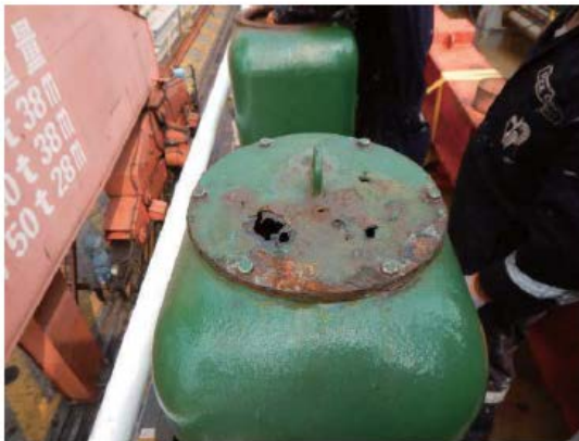
Corrosion holes in air pipe head
