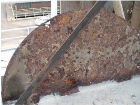
Wastage/Corrosion holes in fire damper flap
