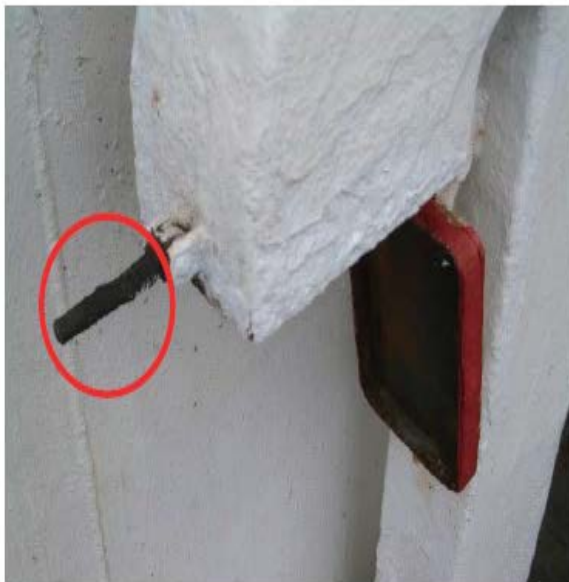
Missing butterfly nut of gooseneck ventilator
