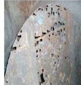
Holes / heavy corrosion on damper housing and flaps
