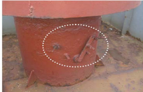
No marking of "Open-Shut"
