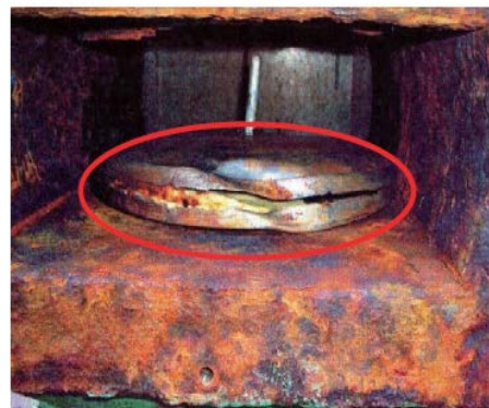
Damage of disk float
