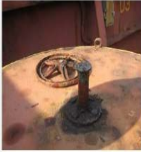
Operating handles not in good working condition
