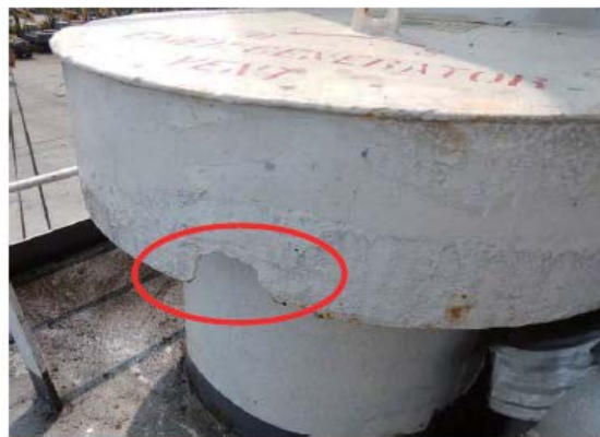
Wastage of the casing of ventilator
