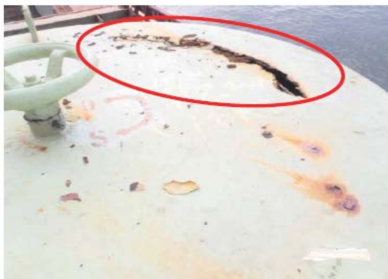
Corrosion holes in the casing of ventilator
